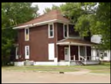
Dilapidated, vacant structures scattered throughout the neighborhood not only constitute a nuisance, but also pose a threat to the health, safety, and welfare of other properties in the neighborhood.
