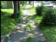
Dilapidated sidewalks need to be repaired in order to make the neighborhood more pedestrian friendly.
