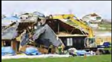
Trackhoe tearing down a house. One idea in this plan is creating a salvage yard of historic materials to reuse in the neighborhood.
